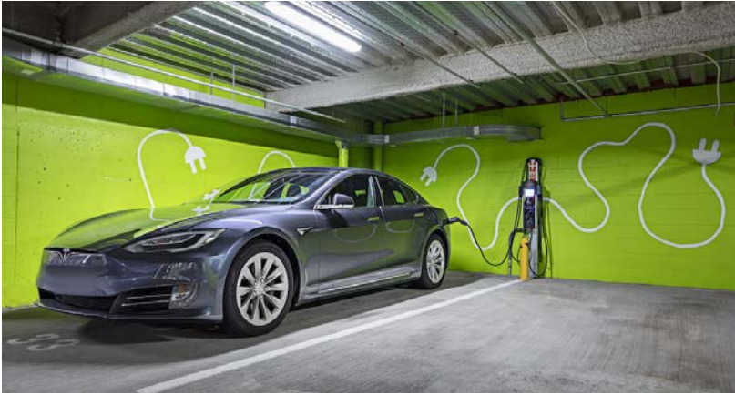
Electrical Vehicle charging in parking garage
