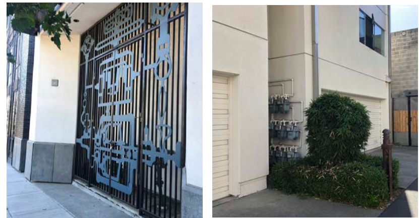
Ideally, utility boxes are screened or hidden behind landscaping or architectural screening.
